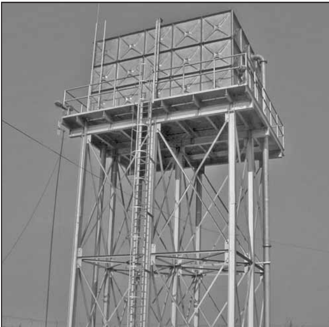
Fig. 1. Overhead water storage tank at Kanyama Water Trust offices
